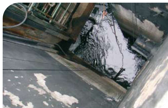
ViSolid and VisoTurb sensors installed in a clearwell to monitor the plant's effluent.
